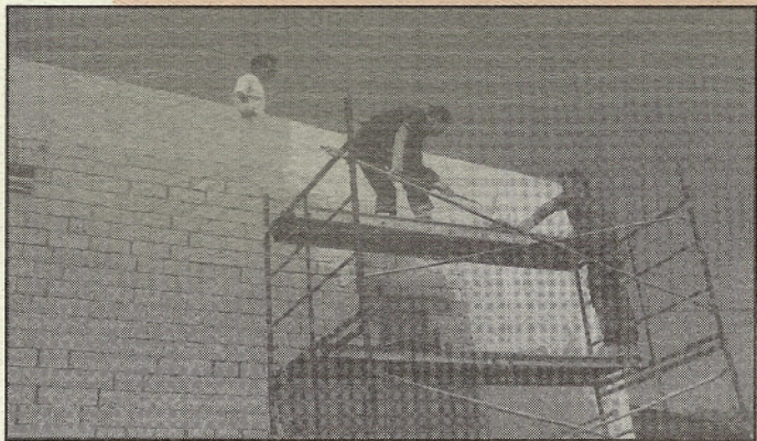
Figure 2. Application of composite fabrics to the URM wall (Courtesy of Structural Rehabilitation Corporation)
